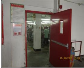
Photo of fire safety equipment Fire door.JPG
