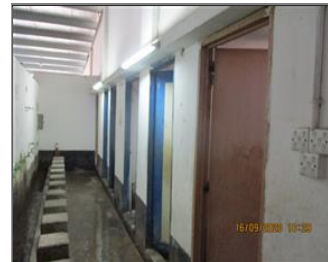
Photo of the sanitary facilities Workers Toilet area.JPG
