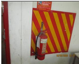
Photo of fire safety equipment Fire extinguisher.JPG
